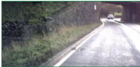
A682 southbound – unprotected bridge pier
