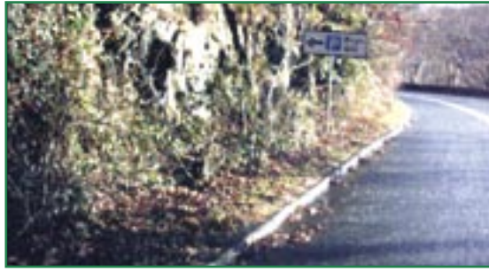
A5 Bangor to A494 eastbound. Poor-run off score - vertical rock face
