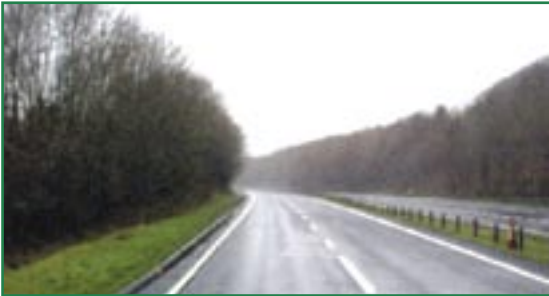
A40 Carmarthen to St. Clears. Poor run-off score due to tree line
